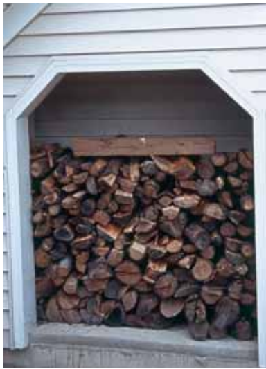
Keeping firewood close to your home is an unsafe practice. It increases the risk of fire spreading into the home.
